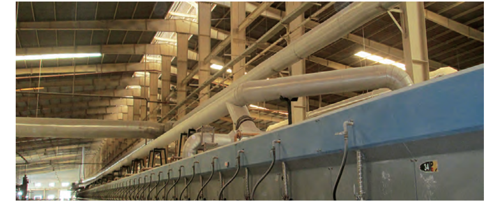
Dust Collection and Raw Material Recycle System / 中央集塵系統
